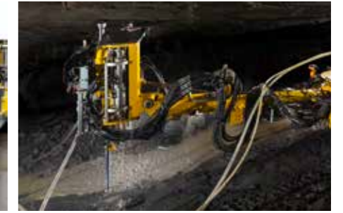
Cabletec SL drills a hole diameter of 38 mm using fully mechanized extension drilling up to 6 m hole depth.
